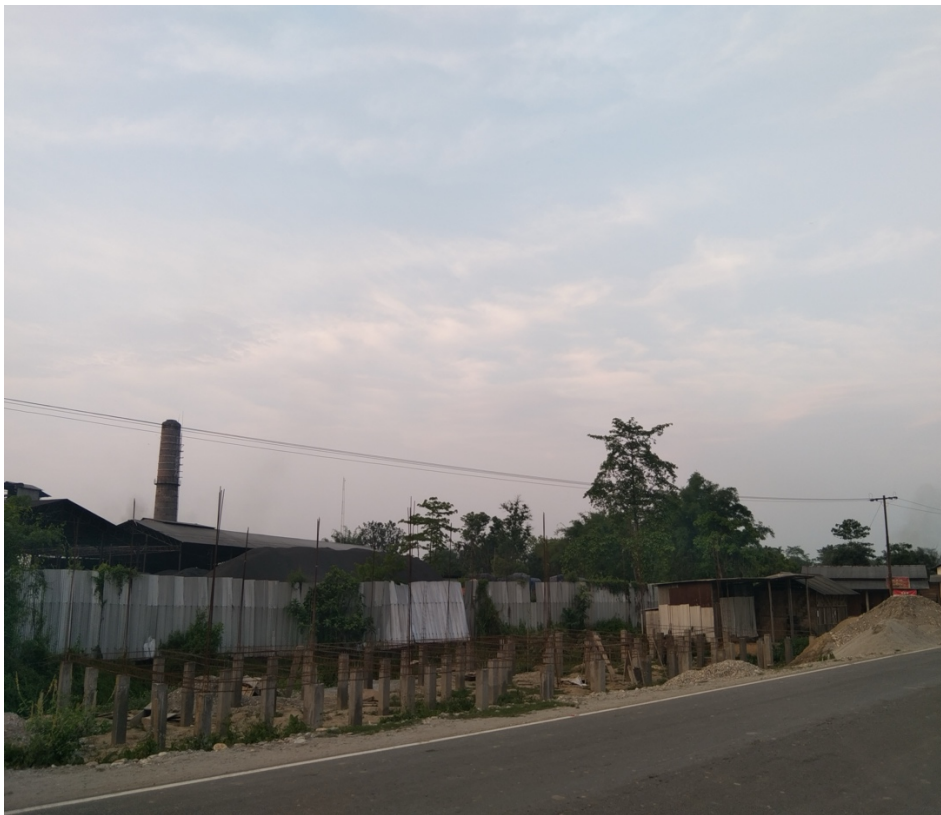
Under construction Shops in front of a Coke plant at Balinong Chariali, Kharsang
